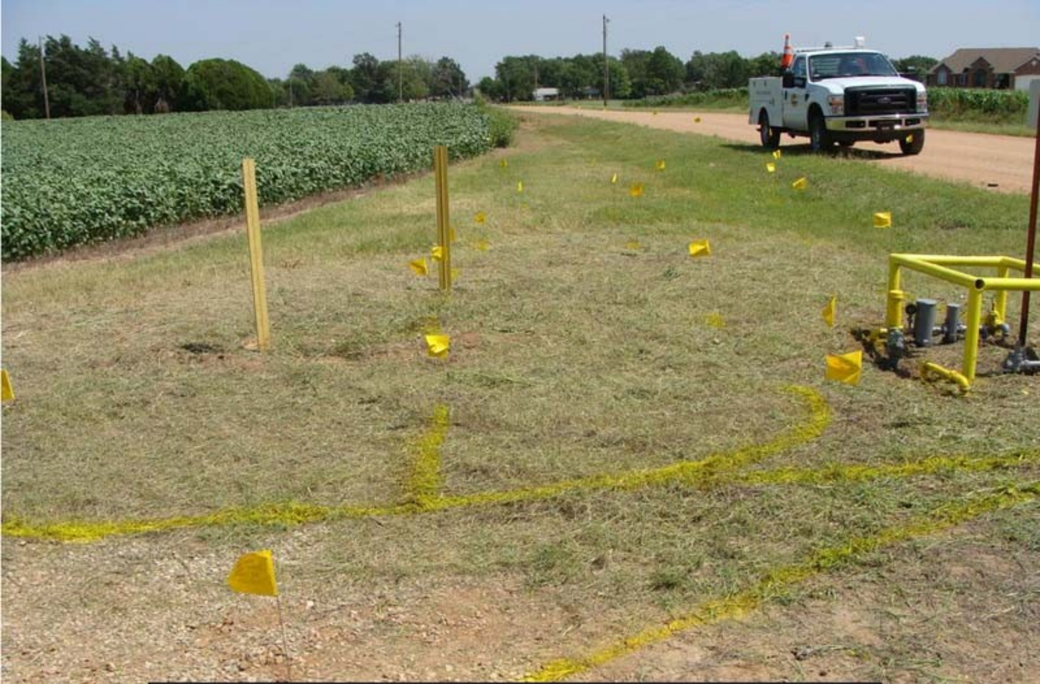
Locating gas facilities near TBS
